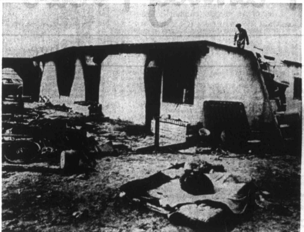
THREE CHILDREN KILLED — Fire Marshal Joe Wilson climbs onto the roof of the de la Rosa family home in El Paso where three children died Tuesday night in a fire. They were identified as Cruz, 1; Daniel, 5; and Petra, 10. Wilson blamed the fire on faulty electrical wiring and said firefighters were hampered because the abode home is four miles beyond any public water lines. Four children were injured, including two who were hospitalized in critical condition. (AP Laserphoto)
