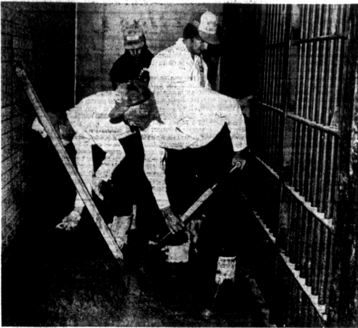
FINAL POUR — Employees of H.R. Bundock General Contractor were busy this morning spreading concrete topping on the final portion of floors in the new county jail. Today's effort
