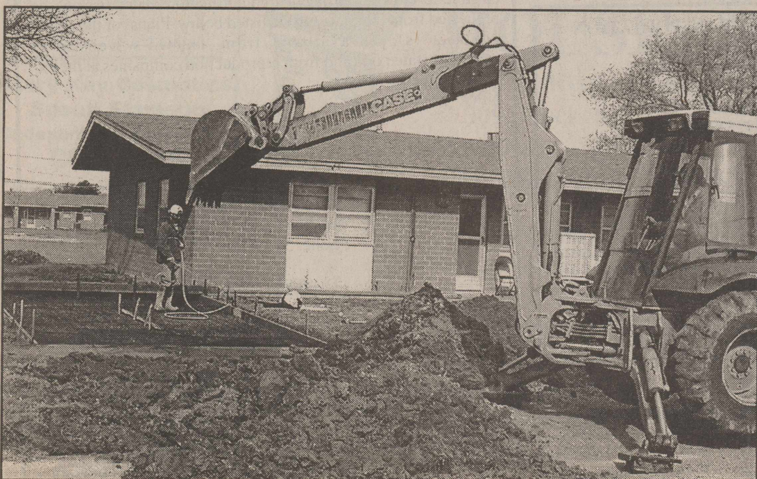
FLOYDADA HOUSING AUTHORITY MAKING IMPROVEMENTS-Monday morning the Floydada Housing Authority was making driveway improvements at 500 E. Clover. Trees were also being planted at the Duncan Apartments, according to FHA Manager Sudy Cochran.
