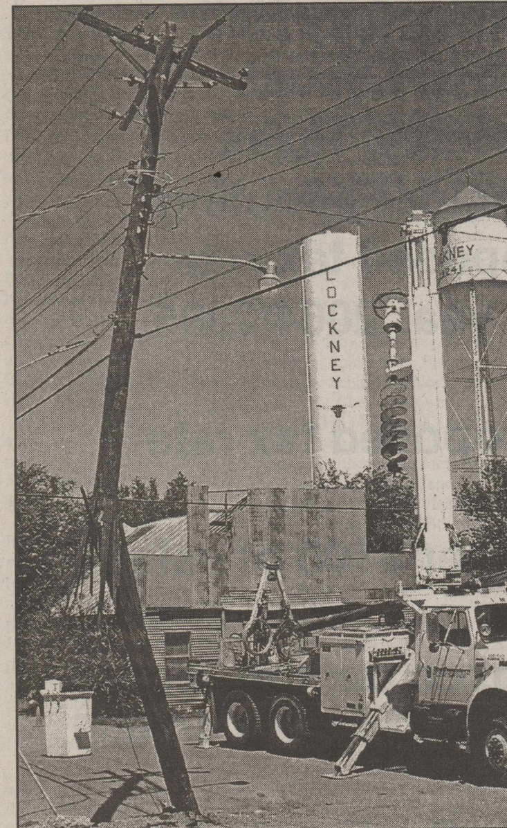
UTILITY POLE snapped Thursday just north of Allsup's on Main Street. A tractor trailer rig turned too sharply and hit it according to the clerk inside at the time. Staff Photo
