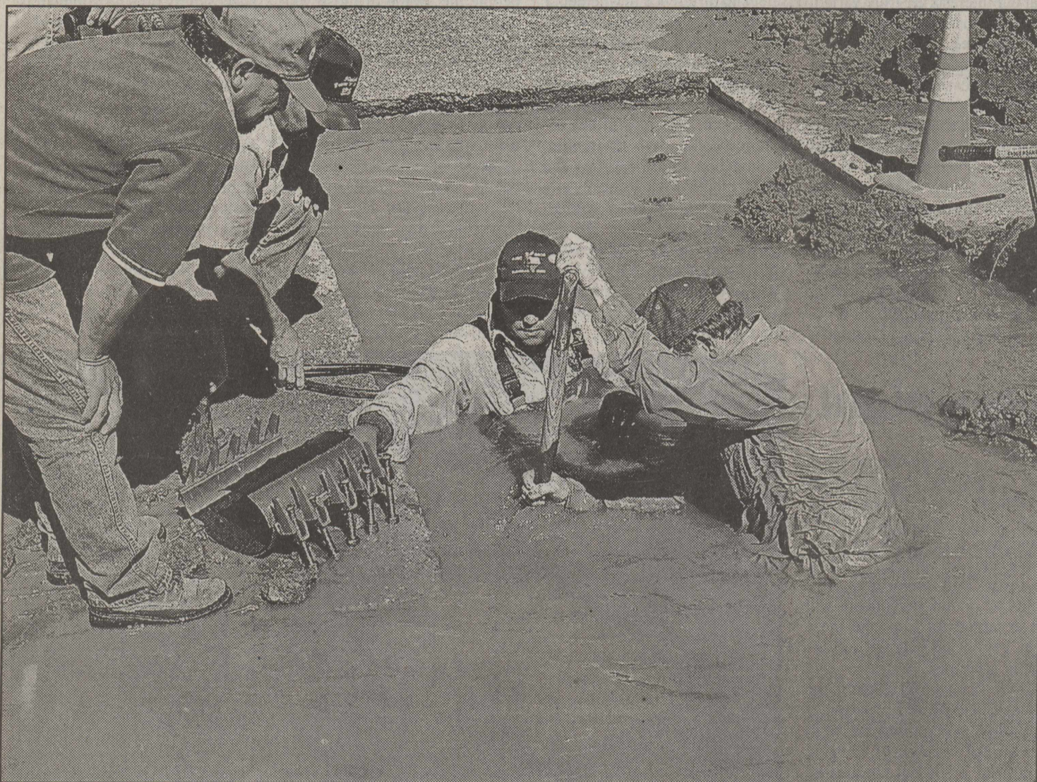
REPAIRING WATER LINE BREAK --City of Floydada Water Department workers were up to their necks at times while repairing this 4 inch water line break in Floydada, Wednesday, October 22, on California Street. Shown here are Roel Cisneros (left) and Gary Fuller (right) feeling their way with shovels and by hand through the muddy water in search of the break point.
