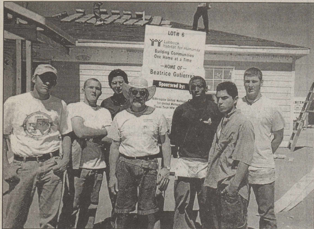
FHS BUILDING TRADES CLASS students donated their time and energy last week to help build a "Habitat for Humanity" home in Lubbock. Students putting their skills to use were: (l-r) Cody Ware, Josh Hammons, Jose DeLeon, Pat Ginn (a former Floydada resident and 1961 FHS graduate), Gerald Henderson, Pablo Salinas, and D.J. Summers. Courtesy Photo
