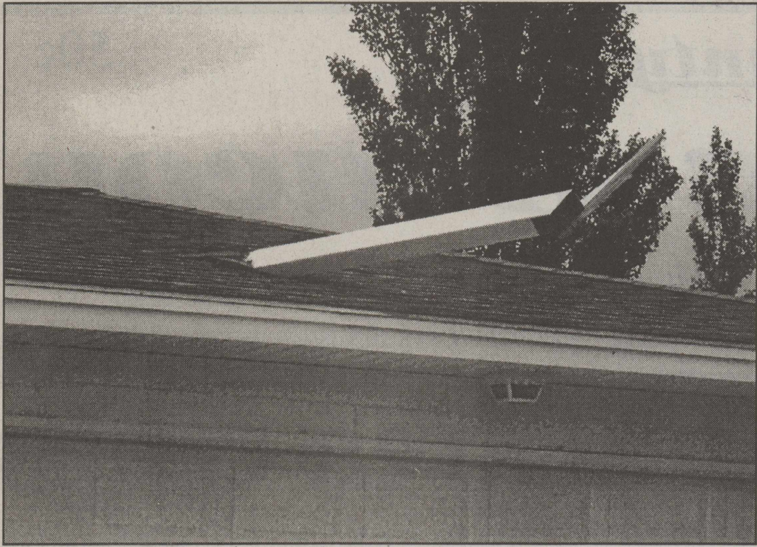
HARD WINDS blew this 4 X 6 pole through the roof of Naomi Johnston, on Apogee Street in Lockney, the night of June 4. Because the direction of the winds were from the north and the pole was driven into the south side of the roof some believe a tornado may have been responsible for the damage. Other poles were spread like matchsticks in the front yard and the roof of the building that was attached to these poles was found across the street.
