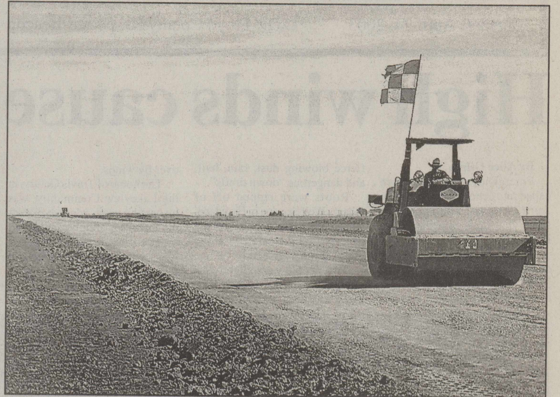
AIRPORT RENOVATIONS NOW IN PROGRESS AS SEEN IN TOP AND BOTTOM PHOTO
