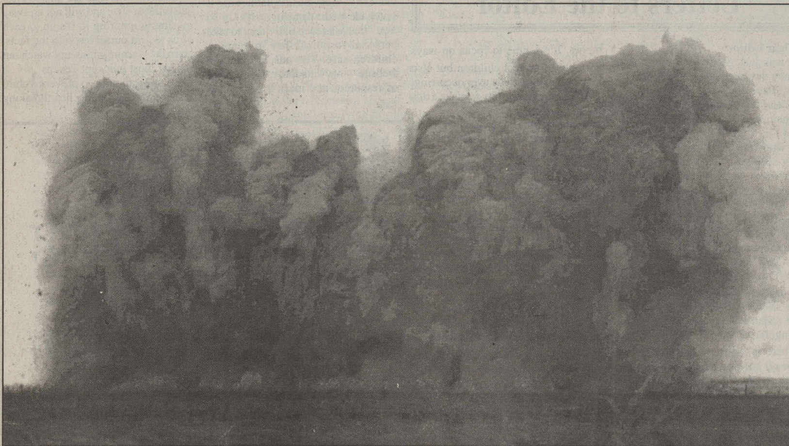
BLASTING AT CALICHE PIT --Martin Morales is in charge of blasting at the Caliche pit east of Lockney. For this blast 127 holes were drilled and then C5 was inserted.
