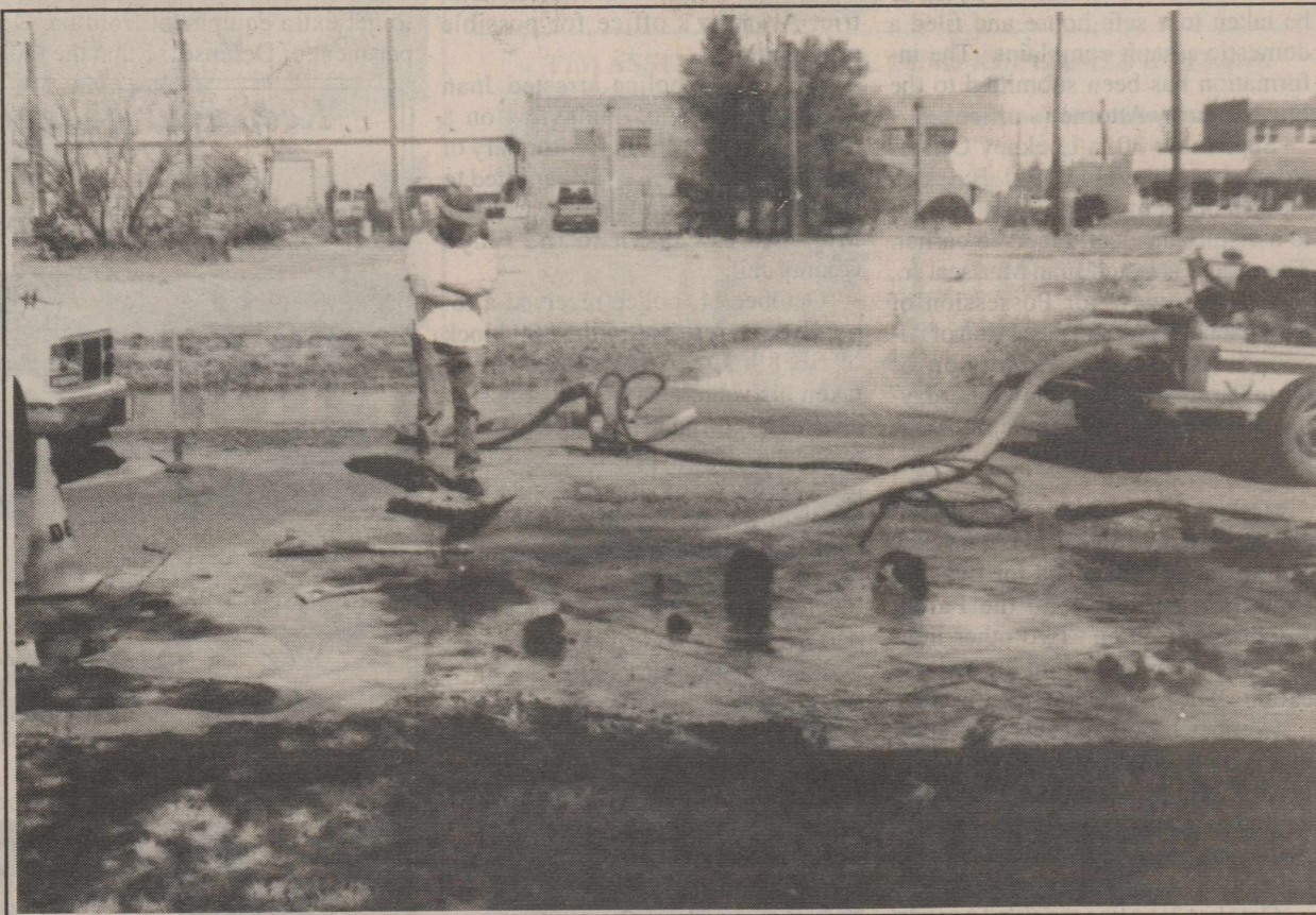
KEEPING YOUR HEAD ABOVE WATER--The heads of city employees (in lower part of photo) are barely visible above water as they worked on the water main break last Wednesday. The water department employees had to repair the line without being able to see what they were doing. Workers worked on the break from 6:30 a.m. until 8:00 p.m.
