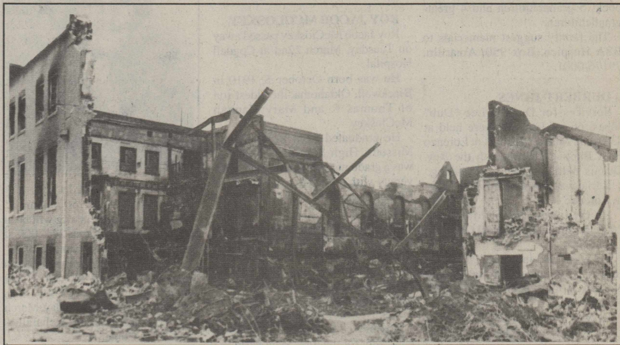
THE WALLS CONTINUE TO BE TORN DOWN AT THE FIRST BAPTIST CHURCH IN FLOYDADA
