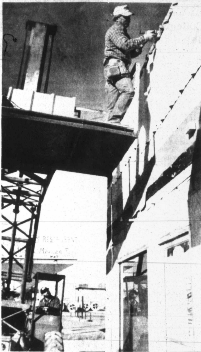
FINISHING TOUCHES — Burton Sandefur puts the finishing touches on the front of the new Radio Shack store while Alan Culp operates the lift. The store is located adjacent to Permian Communications at 2403 25th St. and will be opening Thursday. (SDN Staff Photo)
