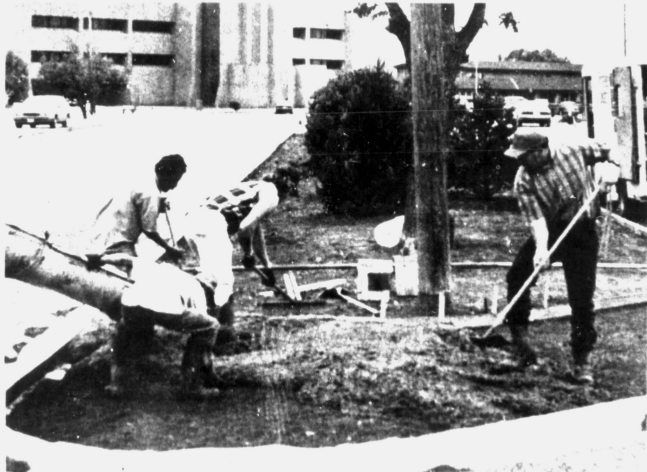
HOSPITAL BEAUTIFICATION PROJECT — Workers with Patterned Concrete of Lubbock begin the final pour on the Rotary Club's beautification project at the entrance to the medical complex. This is the final phase of the project
