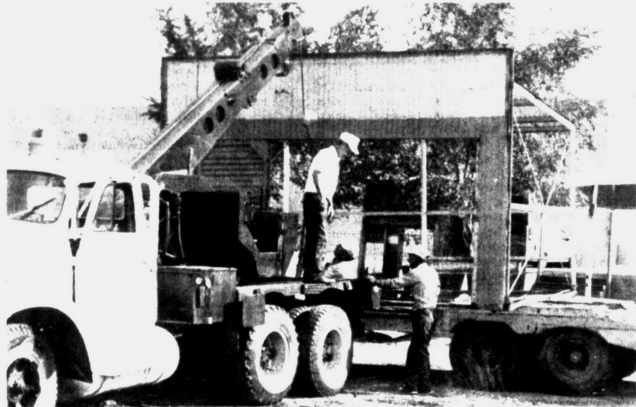
RECYCLING — The city of Snyder is doing its part in the recycling effort as workers prepare to move a building frame from the old Neff Nursery site to the city yard. The structure will be used for storage for tools and materials used in community service projects. City employees loading the frame on a trailer are (left to right) Bobby Kenner, Anson Luna and Wayne Highfield. (SDN Staff Photo)
