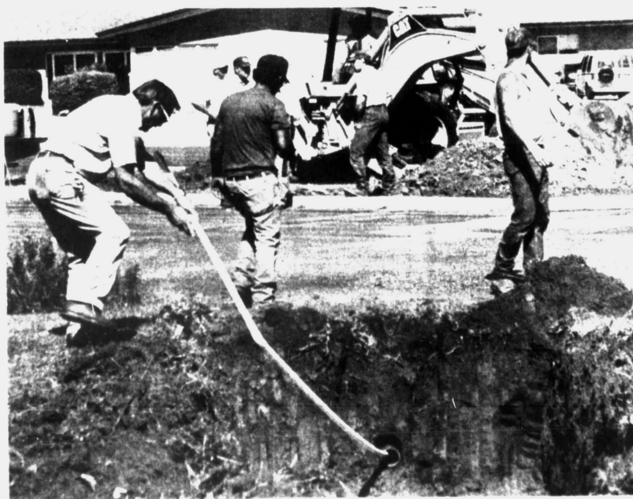
BEAUTIFICATION PROJECT — Cogdell Memorial Hospital maintenance employee Robbie Glascock inserts plastic pipe to be used for watering the entrance at the medical complex here. The work is part of an extensive Rotary Club beautification project. (SDN Staff Photo)
