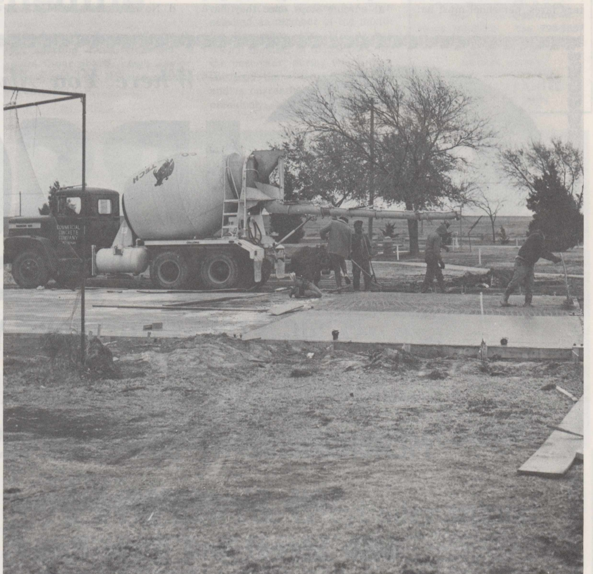
GOLF CARTS —Construction workers are busy pouring cement and preparing the foundation for the new golf cart storage facility located on the North side of the Reese Golf Club. The new brick building will cost $16,864 and is to be completed 120 days after the start of work. This project is one of 11 presently under construction under funds other than Military Construction Projects (MCP) that total $456,984. (U. S. Air Force Photo)
