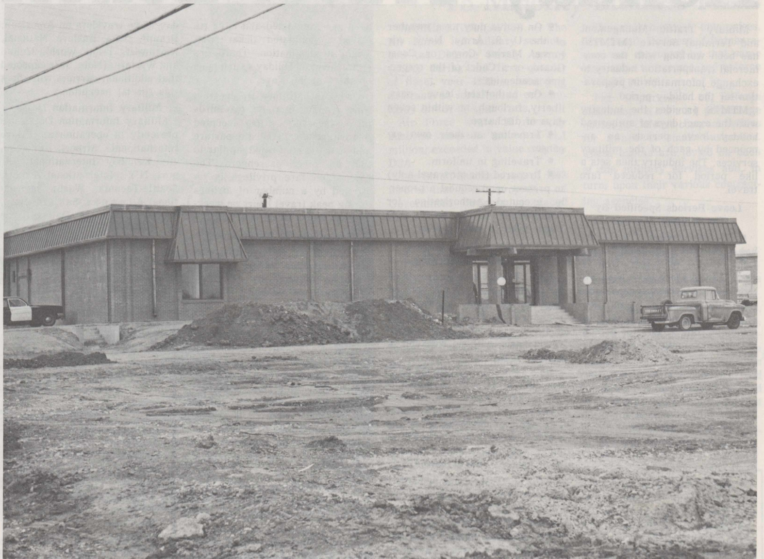
NCO OPEN MESS —The furthest along of the new construction sites, all of which are part of a nearly $1 million Military Construction Project at Reese, is the NCO Open Mess. It is being constructed at a cost of $413,575 and is located at the intersection of 4th Street and "F" Street. The new facility is 80 per cent complete as of Nov. 1 and is due for completion Dec. 15. Occupancy is not expected, however, until early 1972. (U. S. Air Force Photo)
