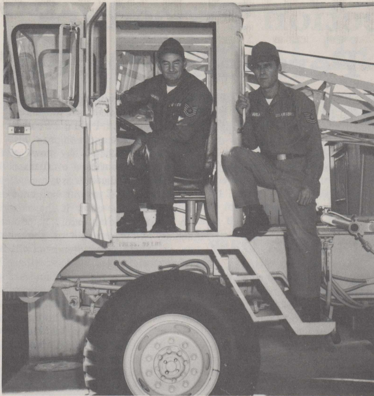
EXPERT RECOVERY—Teihnical Sergeants Horris T. Hamblin, left, and Roberto Davila, both members of the 3500th Field Maintenance Squadron, are pictured with the crane they used to recover a downed helicopter from a cotton field Sept. 3. The two received letters of commendation from Col. Carl L. Brunson, wing commander, for their expert handling of the recovery operation. (U.S. Air Force Photo)
