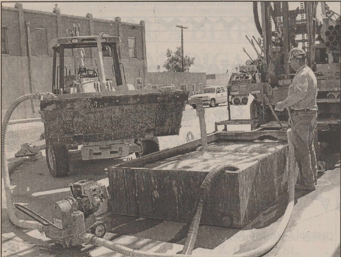
WATER BEING PUMPED OUT, TREATED and reinjected into the water table by way of a recharge well. The rigs and workmen from T & T Drilling of Lubbock were seen at the site of an old filling station at the intersection of Main and Locust streets in Lockney Monday morning, June 19, 2006. T.E.C.Q. required treatment of the currently unused city well to remove traces of benzene. Water quality will be monitored.
