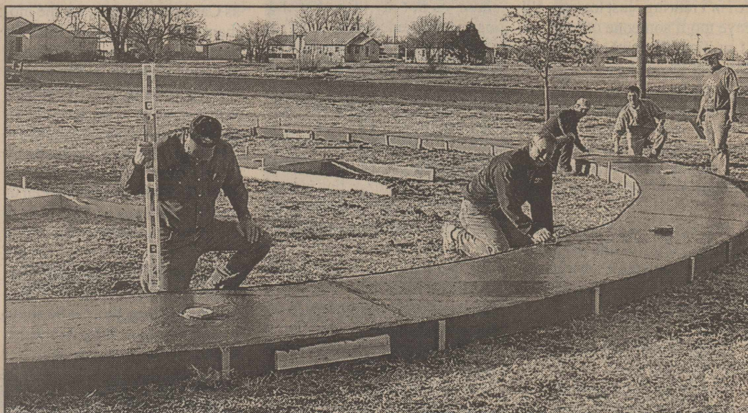
VETERAN'S PARK-- Volunteers lay concrete at the Veteran's Park in Lockney on Saturday. The horse shoe shaped concrete walk will hold Armed Service's flags. They will surround the American and Texas Flags. Donations are still needed to complete the project. Shown here are: (l-r) Ed Marks, Ron Hall, H.G. Graham, Sam Moore, and Dennis Carter. Staff Photo
