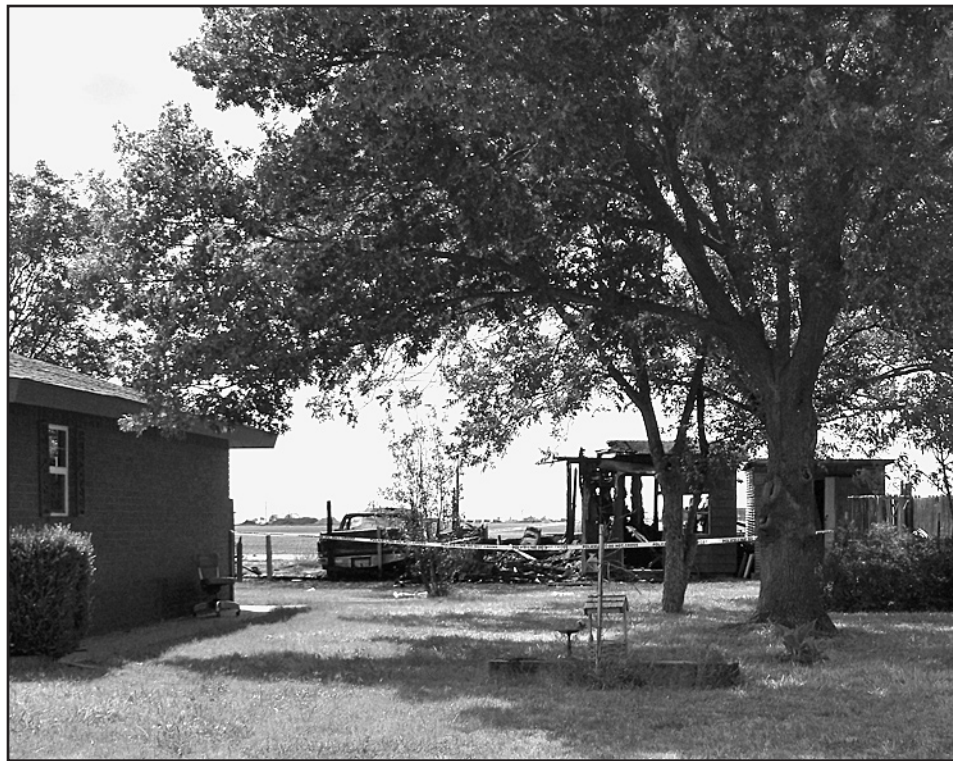
TOTAL LOSS -This storage building at 309 Addison Drive in Haskell was a total loss after a fire late Saturday night, Aug. 27. Haskell volunteer firemen answered the call to find a fully engulfed structure. Police officers and EMS personnel were also on scene. The fire is currently under investigation.
