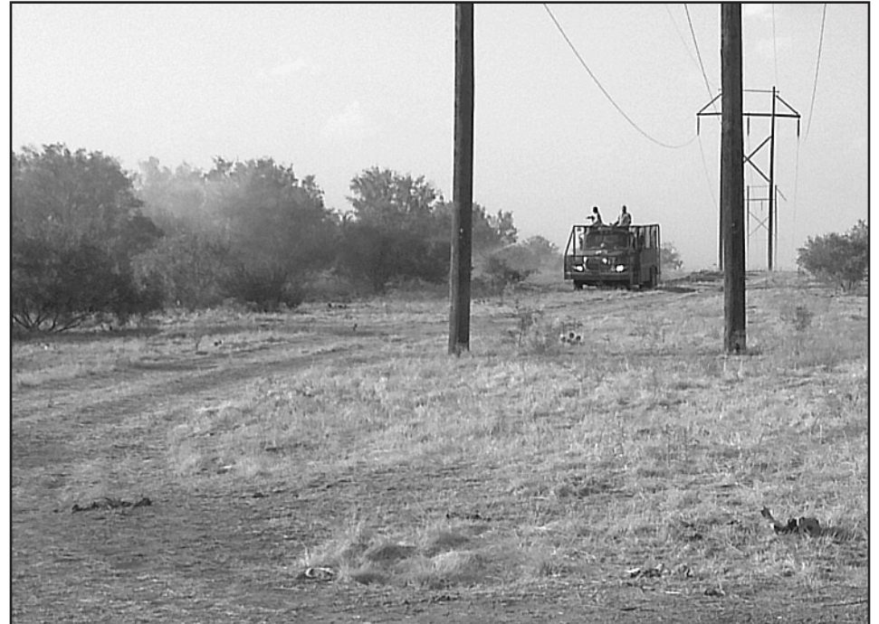
PASTURE FIRE —Haskell volunteer firemen attacked flames on the Hooker Ranch approximately nine miles east of Haskell Fri., Aug. 26. The fire apparently started from an electric transmission line that fell to the ground when the cross arm on the pole broke. Several acres were burned. Fire crews worked into the night to put out the fire.
