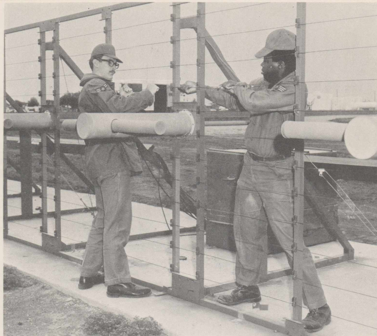
SYSTEM OVERHAUL—ATC Harold P. Johnson, at left, and Sgt. Cleveland Edwards, both of the 2053rd Communications Squadron, install cables during a recent overhaul of the Reese instrument landing system. See story below. (U.S. Air Force Photo)
