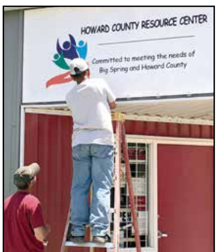
HERALD photo/Anna Gutierrez Workers install a sign May 22 bearing the new name of the Howard County Resource Center, formerly the Northside Community Center, at 110 NE Eighth St.
