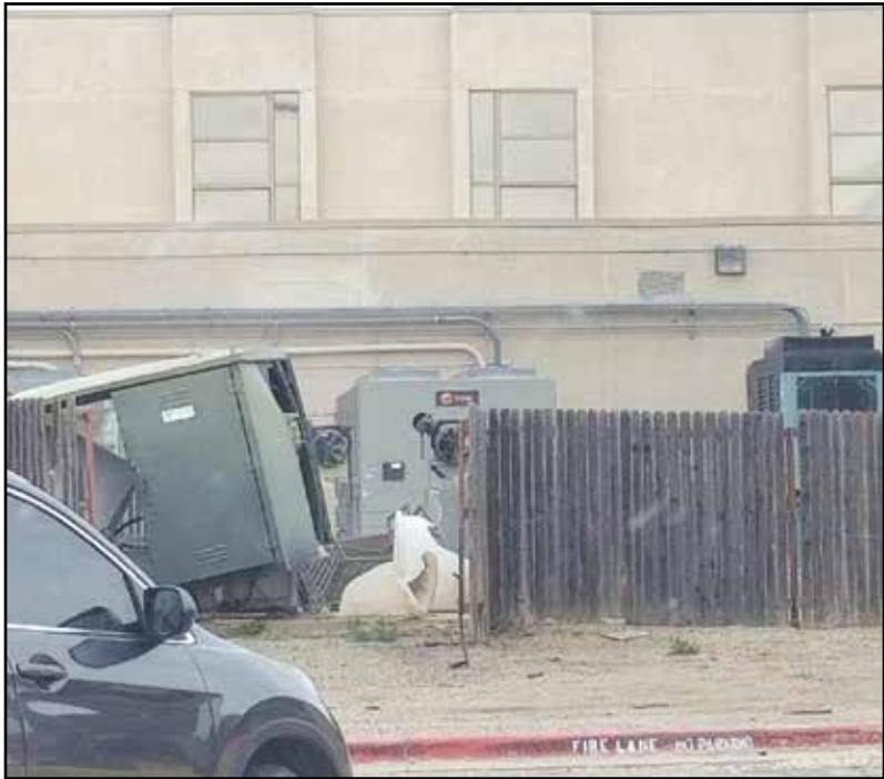
HERALD photo/Amanda Duforat A blown transformer caused a power outage at Scenic Mountain Medical Center and for many local residents Tuesday afternoon. Power at SMMC was expected to be restored today.
