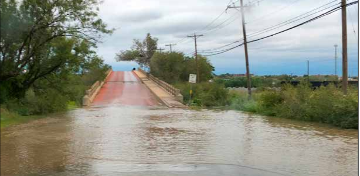
HERALD file photo This photo from Oct. 16 of this year shows flooding caused by Big Spring waterway Beals Creek overflowing its channel due to heavy rain. At its meeting Tuesday, the Big Spring City Council will consider granting permission to go out for bids on a project to rehabilitate construction on the creek's channel. The meeting will be at 5:30 p.m. Tuesday in the City Council Chambers, 307 E. Fourth St.
