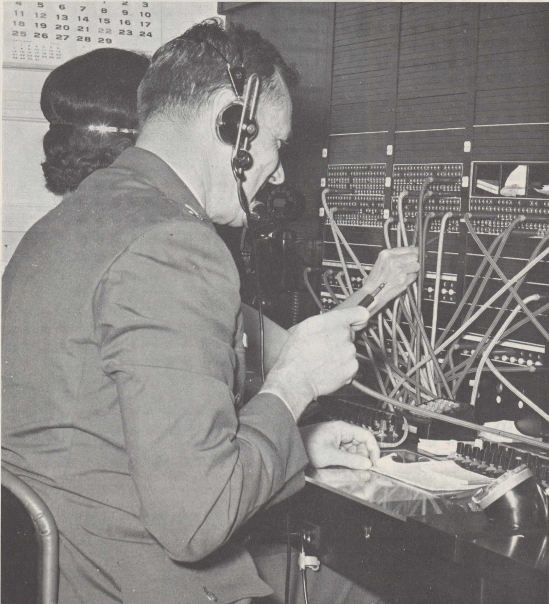
NEW SWITCHBOARD INSTALLED—Col. Clyde J. Morganti gets ready to plug into the new switchboard to officially open it. (AIR FORCE PHOTO By SSgt. Larry B. Hawkins)
