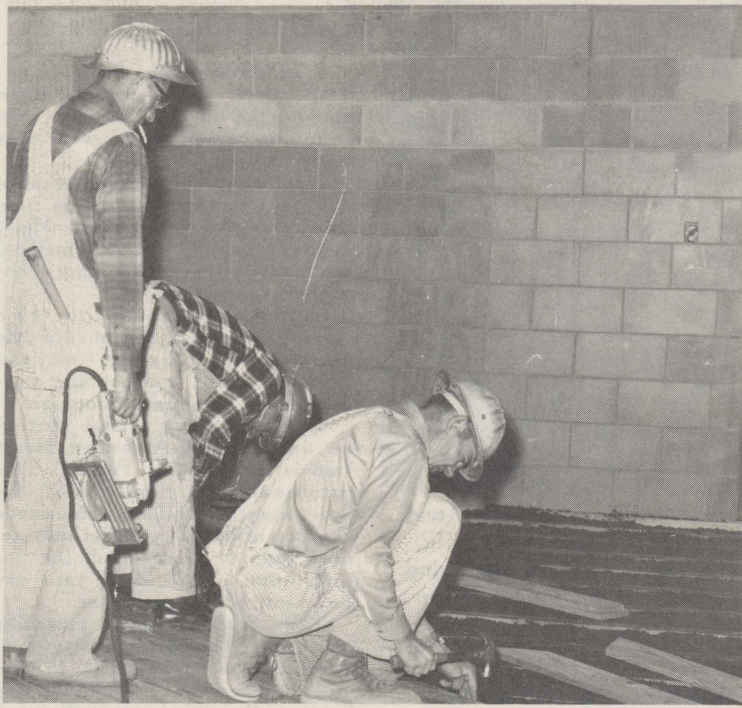
NEARING COMPLETION—Workmen of the C. M. Pharr Construction Co. of Lubbock lay the floor of the newly constructed gymnasium at Reese. The new facility should be available to all base personnel sometime in March. (AIR FORCE PHOTO)
