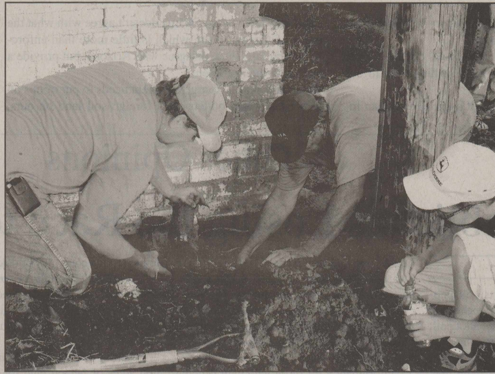
Courtesy Photo Jim Martin and Shad Schlueter are cutting tree roots out of the sewer line at the Fair building. Just three more weeks to get everything in shape.
