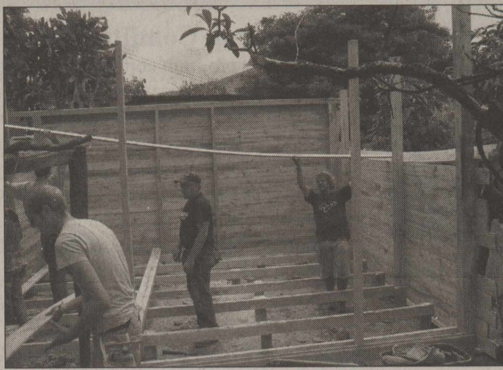
It costs $1,300 to build a home in Honduras and tools consisted of post-hole diggers, hammers and chainsaws. Volunteers, including Childress' Rickey Husband center, built a house for an elderly couple who had lost theirs. (Photos courtesy of Trey Morgan)
