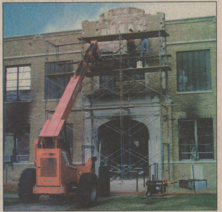
SAVING A PIECE OF HISTORY - Workers removed stonework from the entrance to the burned-out shell of the old Lockney High School last week. The decorative stonework was salvaged for possible incorporation into design of the new LHS building.
