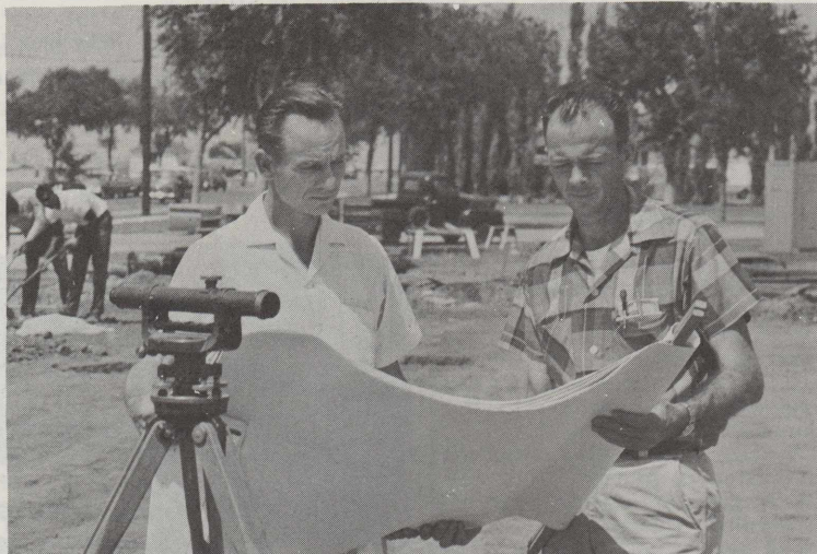
INSPECTING —The Resident engineer, Norval R. Miller, and the base inspector, James A. Goebel, of the Army Engineer Corps' new area office here inspect the plans for the new flight simulator building. Workmen of the W. B. Abbott construction company are in the background. (Photo by Linehan)
