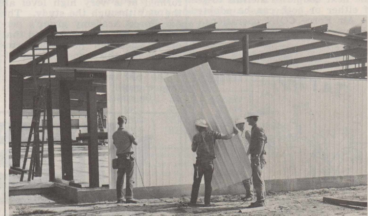
IT WON'T BE LONG—Workmen hoped to be finished today with placing the sides and roof on the new Reese bowling alley. Here they placed a 3 by 8 foot metallic panel on the end wall last Saturday, moving immediately to the sides. The walls and ceiling are insulated and the building is of paneled design, unusual for metallic buildings, officials of the Brown Showcase Co., contractors, stated. Laying of lanes and installation of mechanical equipment, including pin-setters, will be started without delay. (Photo by Roach.)
