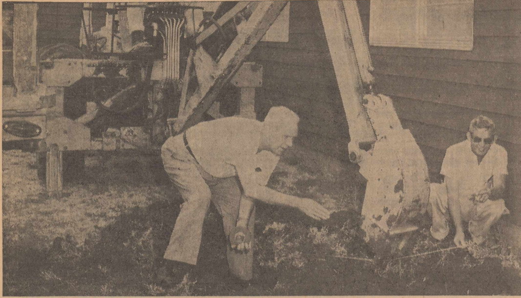
BIG PROJECT STARTS —Work on renovation of units in the Reese housing area is in full sway. The work, to cost more than $944,000, will include enlargement of 417 kitchens, addition of bedrooms to a majority of homes, and general renovation. Here supervisors take a measurement on earth moving as the project
