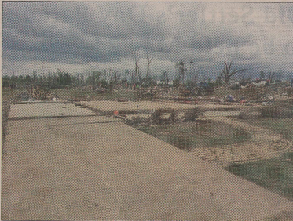
Photo Courtesy of Patty Davenport All that was left of the home of Dennis and Glenna Lavergne was the foundation. Glenna was the sister of Patty Davenport of Floydada. Glenna and Dennis lived in Vilonia, Ark. where an EF4 tornado struck the community and surrounding area killing at least 16 people including the Lavergnes.
