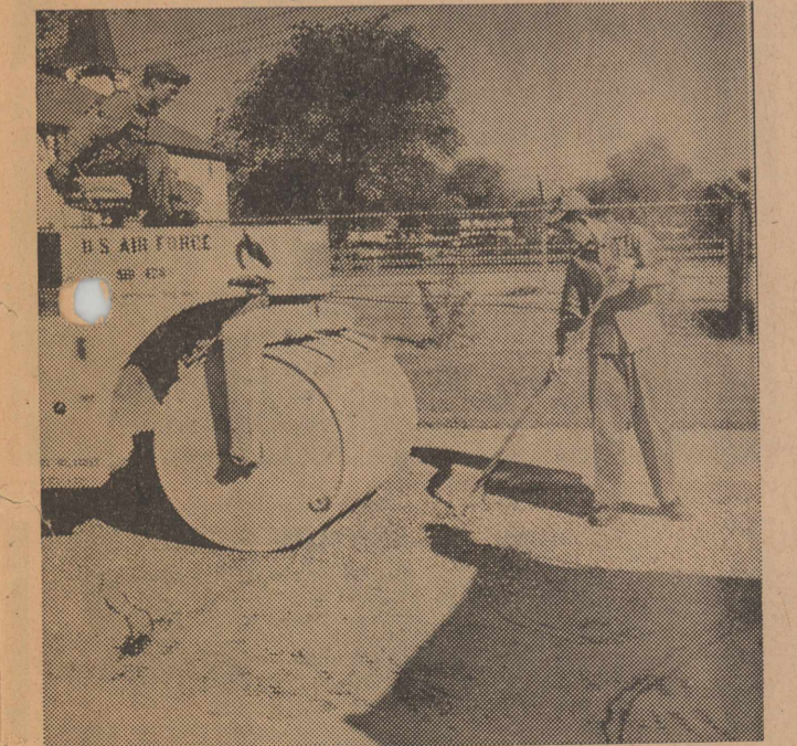
IT'S PACKED —A 10-ton roller packs the street and parking areas firmly. A/3C Eddie Lampp and A/2C Melvin Thrasher are operators.
