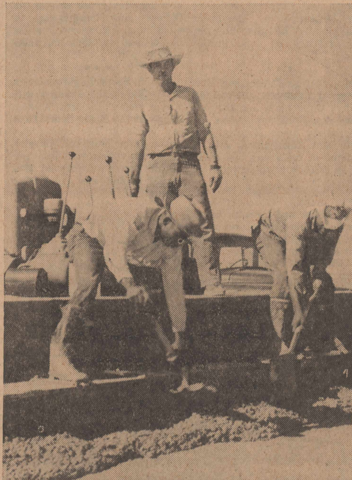
IT MUST BE SOLID —A spreader and vibrator pack the concrete solid on Reese's runway extension. Here workmen add a hand-spread touch to the project while standing on the spreader-vibrator which shakes, packs and distributes the "mud." (Photos by Santangelo)
