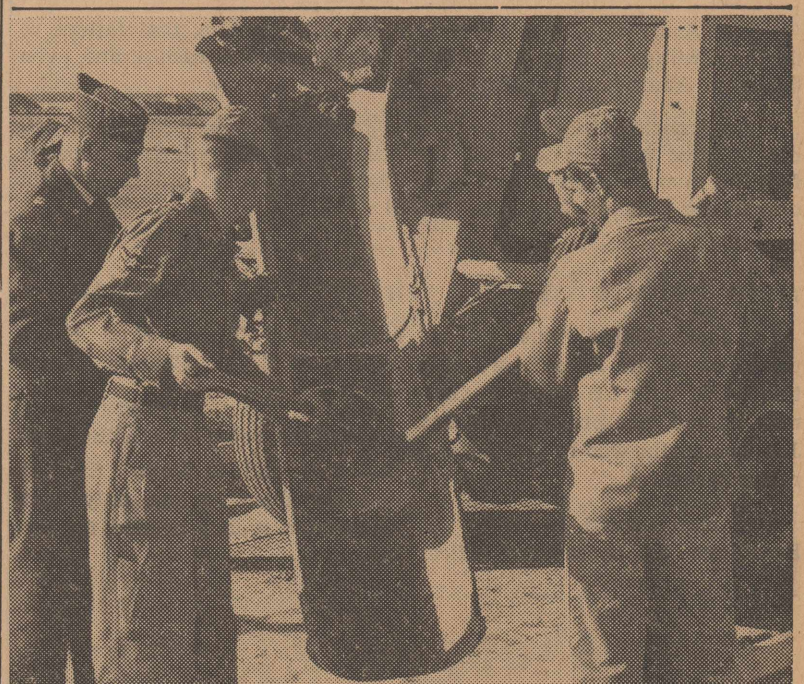
CLUBHOUSE STARTED—Volunteers started work last week on the new Reese golf clubhouse. Shoveling the freshly made concrete for the footings are (left to right) Capt. Frank C. Lee, Installations operations officer; A/3C Karry Graven, volunteer worker; Capt. John Johnson, assistant operations officer, and A/3C Roland Sakall, another volunteer. The clubhouse designs call for a sweptback wing formation. One wing will house the greenskeeper office, a snack bar, restrooms and stockroom and some wall lockers. Another wing will contain lockers beyond the breezeway. Each wing measures 25 by 72 feet. The breezeway will be 25 feet wide in front and 16 feet to the south. (Photo by Roca)
