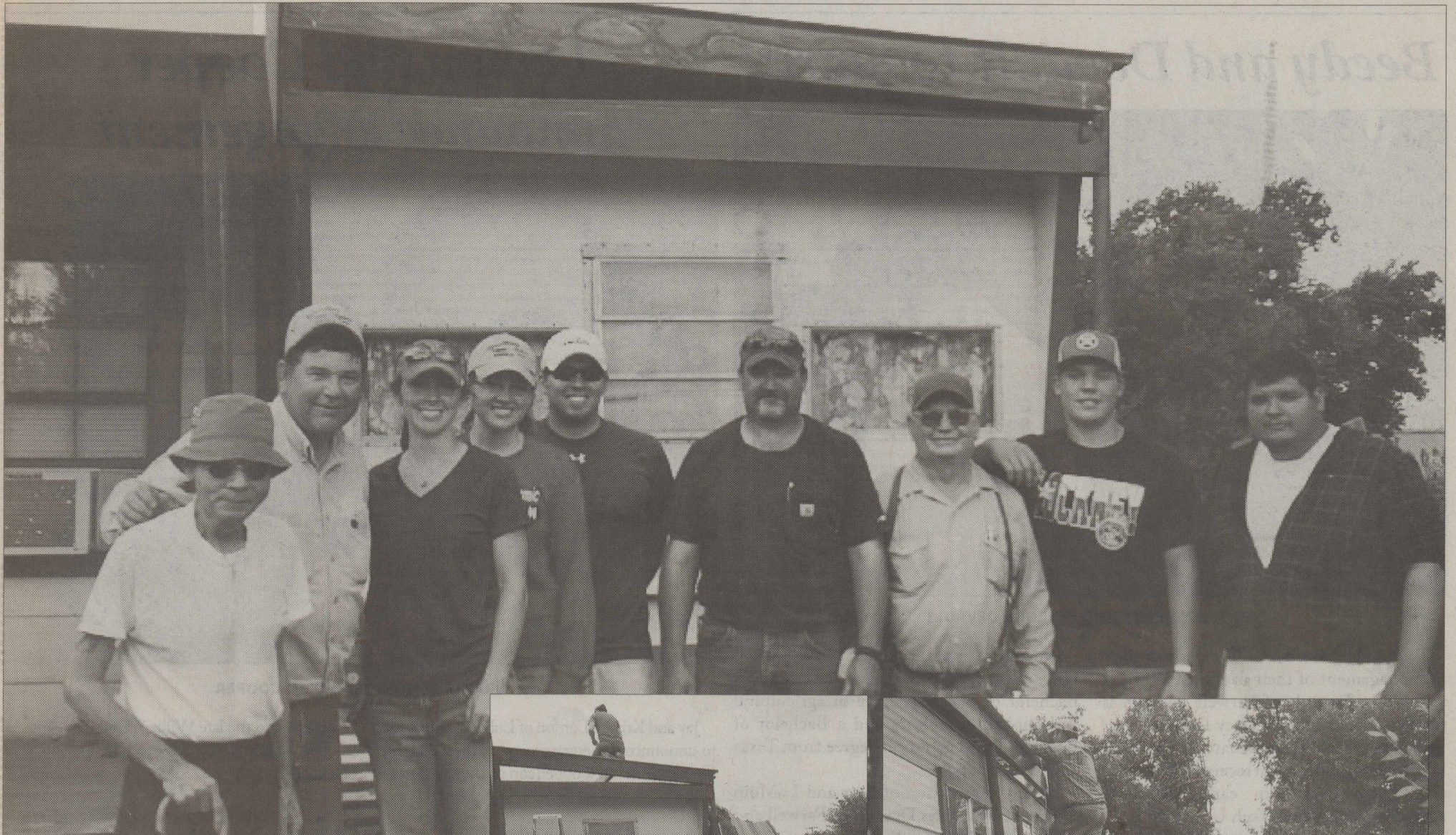
Courtesy Photos Members of the First Baptist Church in Lockney spent a day at the home of Oscar and Teresa Gonzales mending their roof. Mr. Gonzales is undergoing treatments for cancer and was unable to keep repairing the roof.
