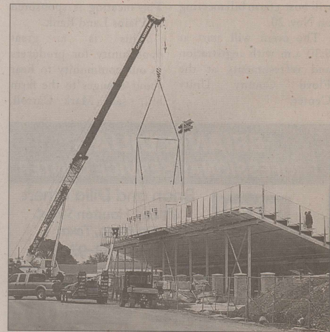
Last Friday, Nov. 8, the press box was lifted in place at the new Whirlwind football field. New drone pictures of the progress of the new stadium and school will be in the upcoming issues.
