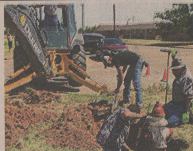
Lockney's Public Works crew replaces a fire hydrant on North Main last year. CDBG funding should allow for additional equipment upgrades this year.
