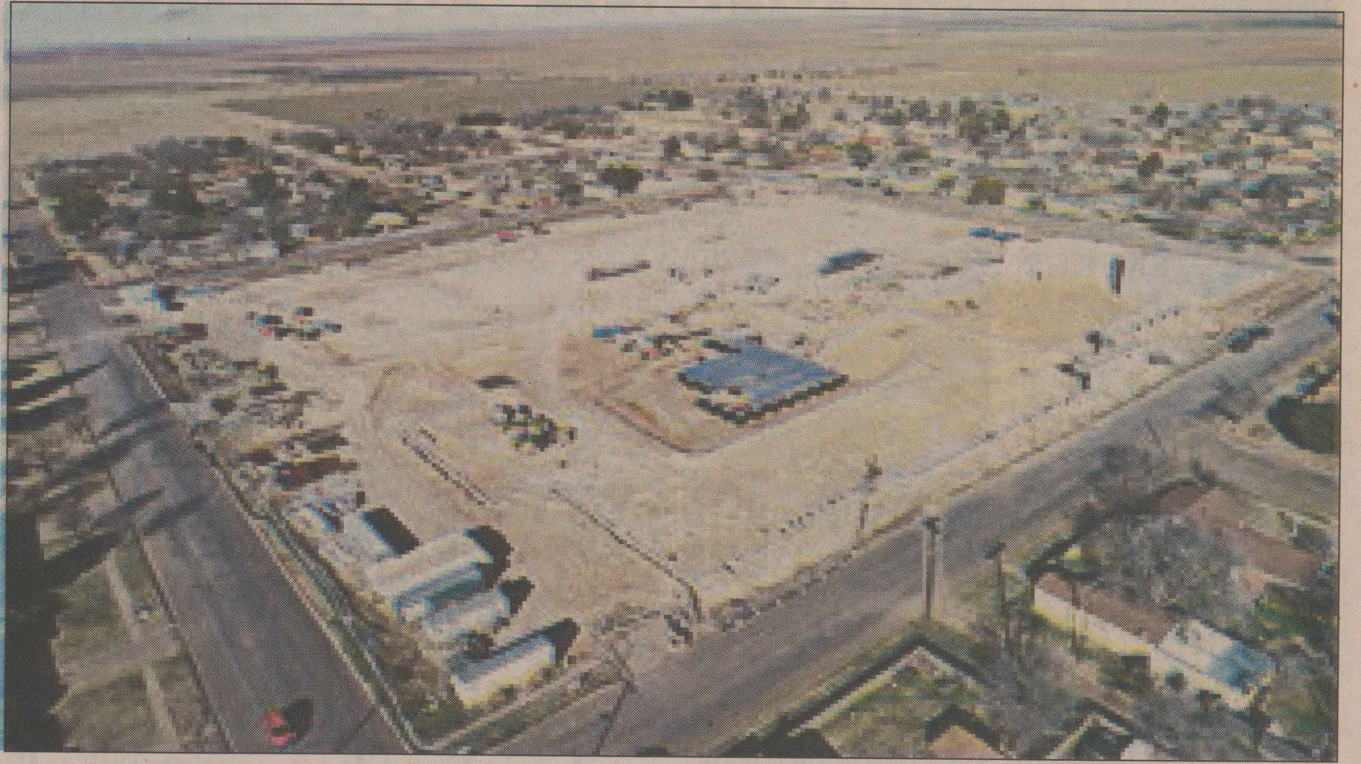
Aerial view of the construction site looking from the southeast to the northwest.
