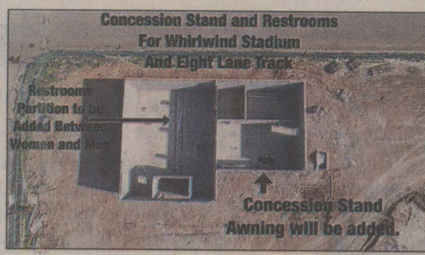
The concession stand and restrooms for Whirlwind Field and Track are shown in the three photos pictured above. Once crews are on site to begin placing structural steel the roof will be placed. The concession stand is on the right side of the building and will have a covered awning over the serving windows. The wall between the men and women's side will be built when the roof is placed. The building has block walls now but will be bricked to match the construction of the high school, CTE, band hall, and auditorium when they are completed.
