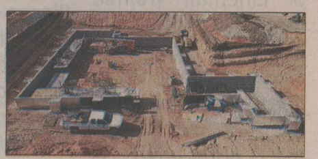
public. Beginning in the next few weeks, the wall and structural steel for all of the main buildings will start going up which will allow the public to actually see progress.
