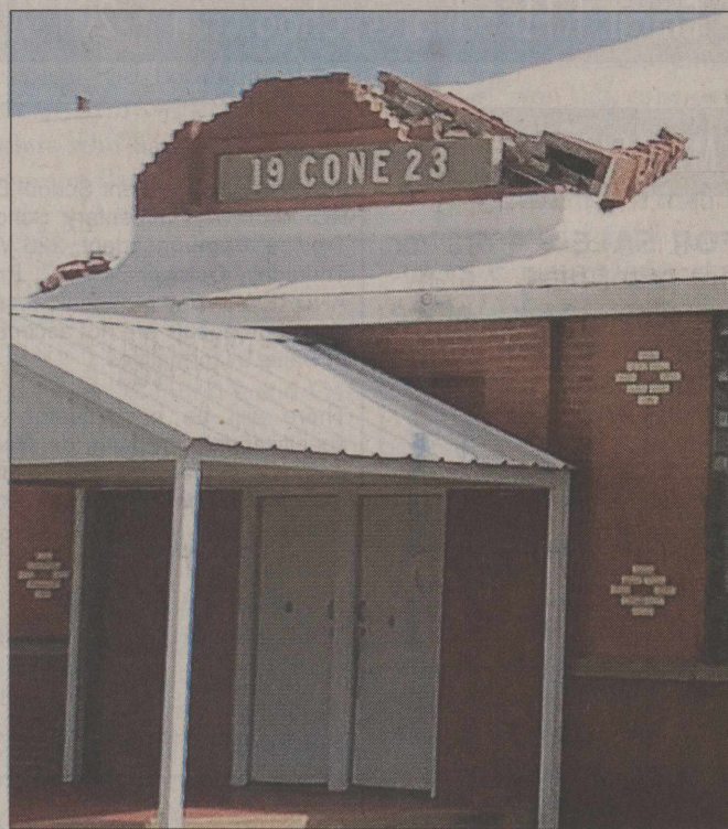
The historic Harmony Plains Singing School was damaged by a storm Sunday night. Many structures in Cone suffered wind damage.
