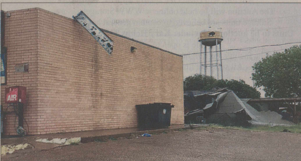
Sunday night winds reported at 60 to 90 miles per hour blew the roof off the Petersburg Allsup's onto another house. Similar damage was reported from the storm in Cone.
