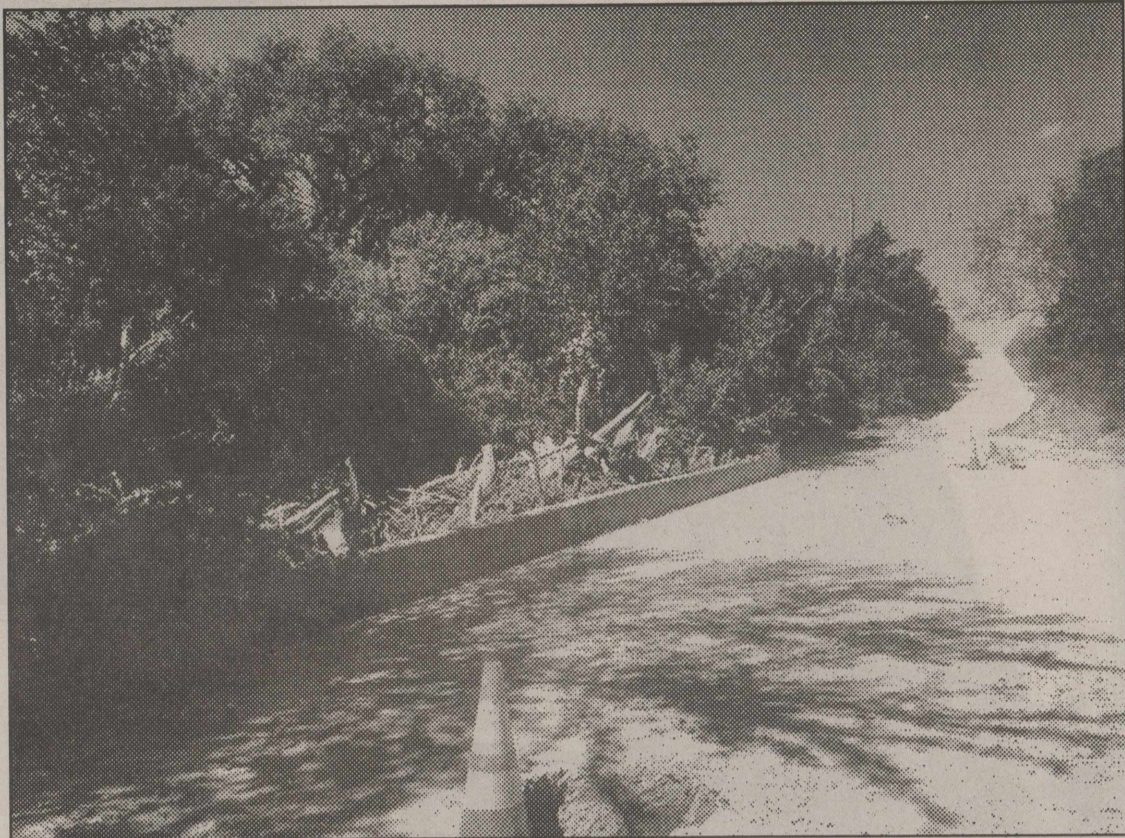
Damage! Mid-September rains led to this bridge on Ross Road in northern Coke County being damaged and closed. Coke County Precinct 2 had been working on it prior to these most recent heavy rains.
