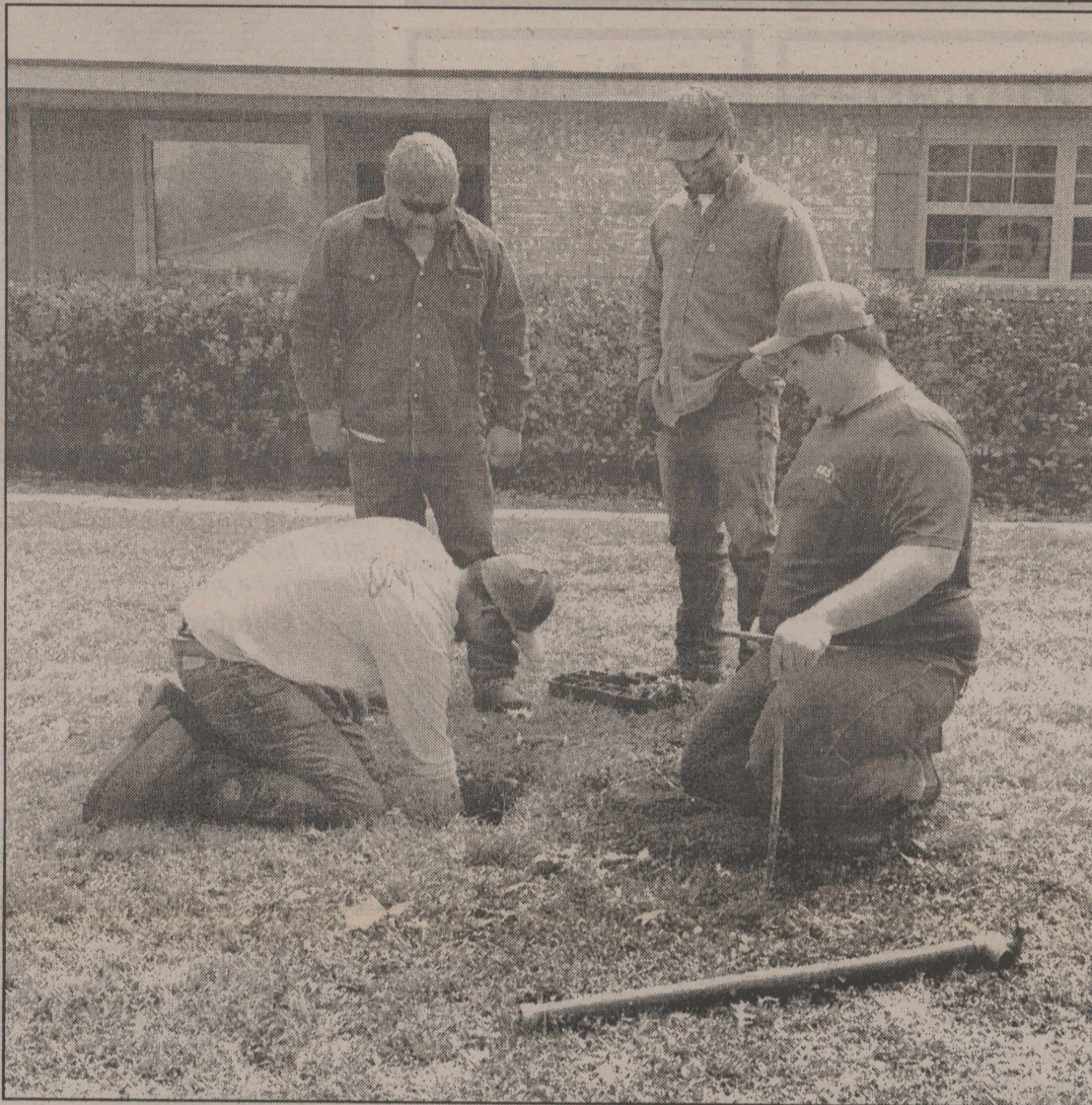
New Water Meters! In the next week or so if you see Robert Lee city workers and others working in yards and alleys, they are replacing the old water meters with new digital meters. The new program is the result of a 70/30 grant received by the City of Robert Lee for this purpose.
