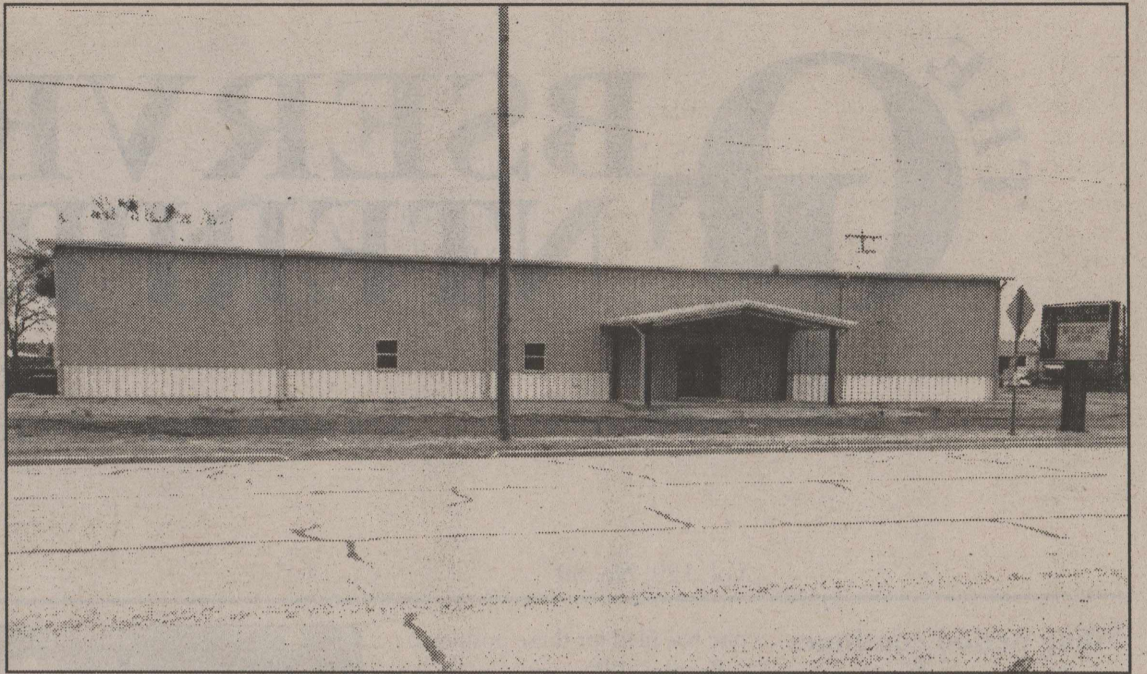
New Church Building! The new activity center for First United Methodist Church in Robert Lee is coming along nicely. Construction of the center should be completed in March of this year.
