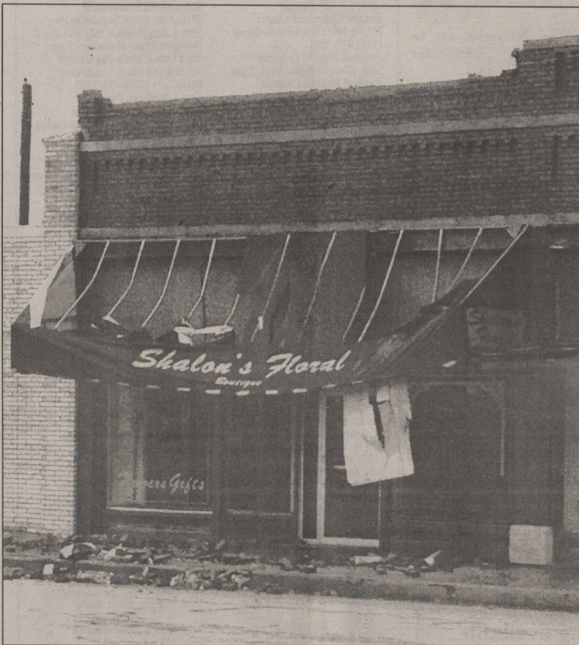
Storm Damage! Last week, another storm came through and proved to be the final straw for this awning in downtown Bronte.
