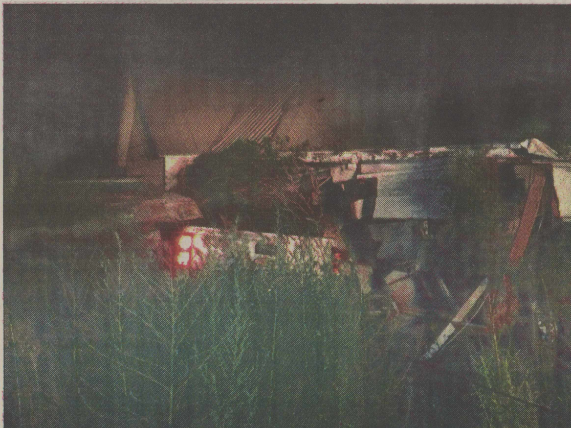
House Damaged! At approximately 2:40 am Saturday morning, July 25, 2015, a pickup crashed into the home at 1010 Austin Street in Robert Lee. The driver of the pickup is from Snyder and while traveling northbound on State Highway 208, failed to negotiate the curve on State Highway 208 just past the State Highway 158 intersection. The driver was arrested for driving while intoxicated by DPS Trooper Dykstra. Also assisting with the accident were Coke County Chief Deputy Brandon Neal and Deputy Terry Crenshaw. A resident of the home was taken by ambulance to the hospital, but was treated and released.
