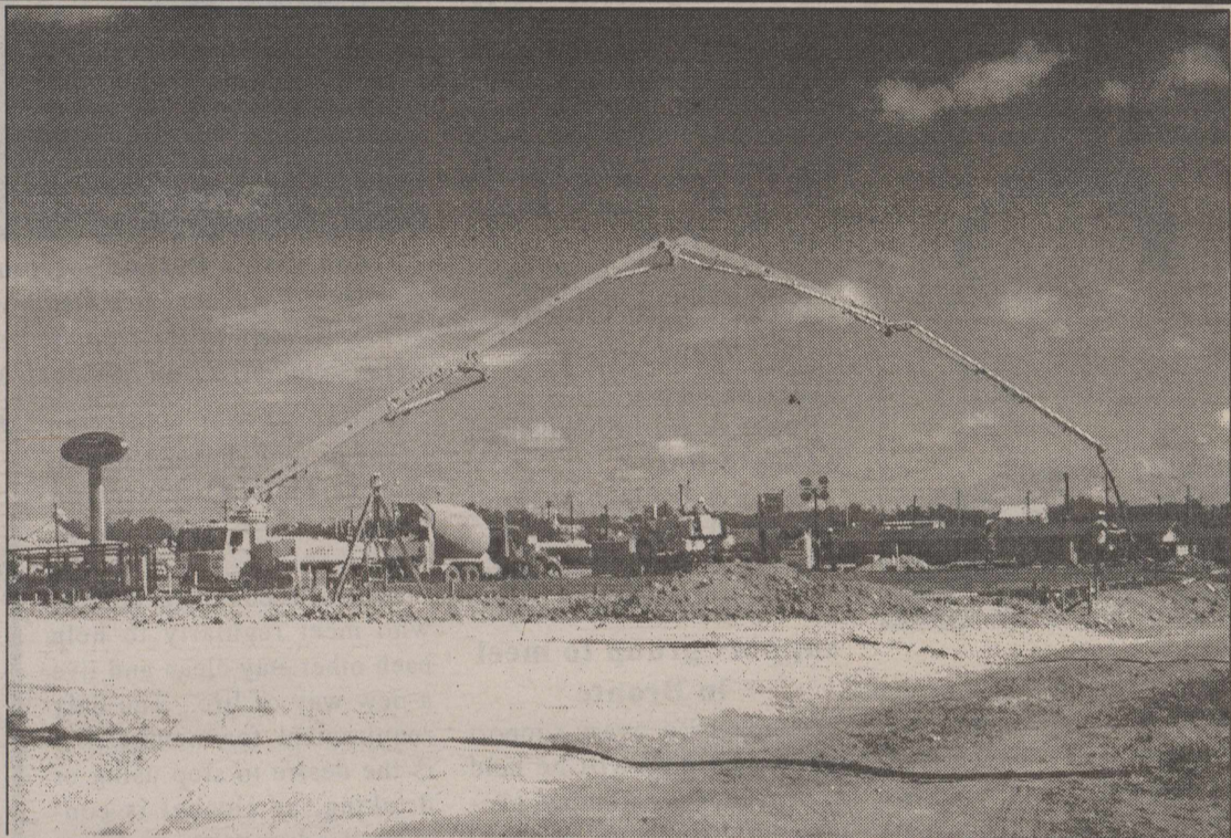
Signs of Progress! It's readily apparent when you drive down Commerce Street in Robert Lee that the new Family Dollar store is coming soon. The foundation was poured for the new store Monday morning, September 9, 2013.
