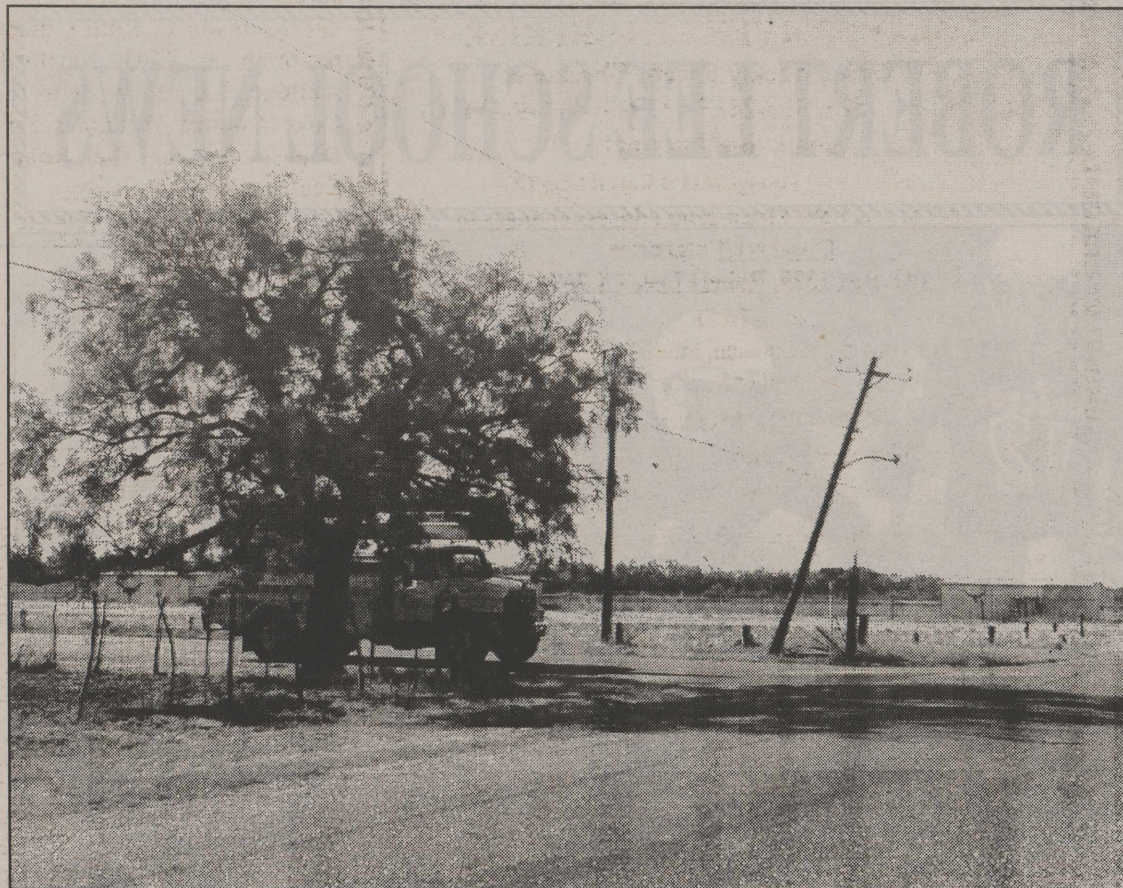
Broken Utility Pole! Someone broke this utility pole in the 600 block of South Jefferson in Bronte last Thursday morning, August 29, 2013, just after 8 am. Fortunately, no lines were on the ground.
