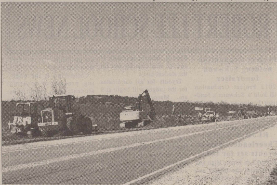
Pipeline Nears Completion! You can see in the photo above, taken Tuesday, March 20, that the two ends of the water pipeline running from Bronte to Robert Lee are only about 100 yards apart. The pumps will not arrive in Robert Lee until April 1, shoving the official completion date back to the middle of April. However, according to city officials, Robert Lee is in no danger of running out of water before the completion of the pipeline and pumping system.
